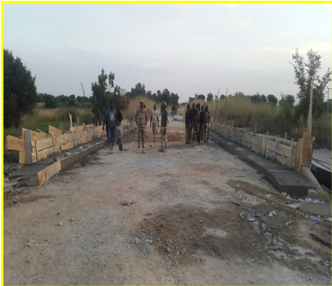
Picture Plate 2: Military Construction of Road Gwoza – Yamtake Bridge Source: Army Public Relations
