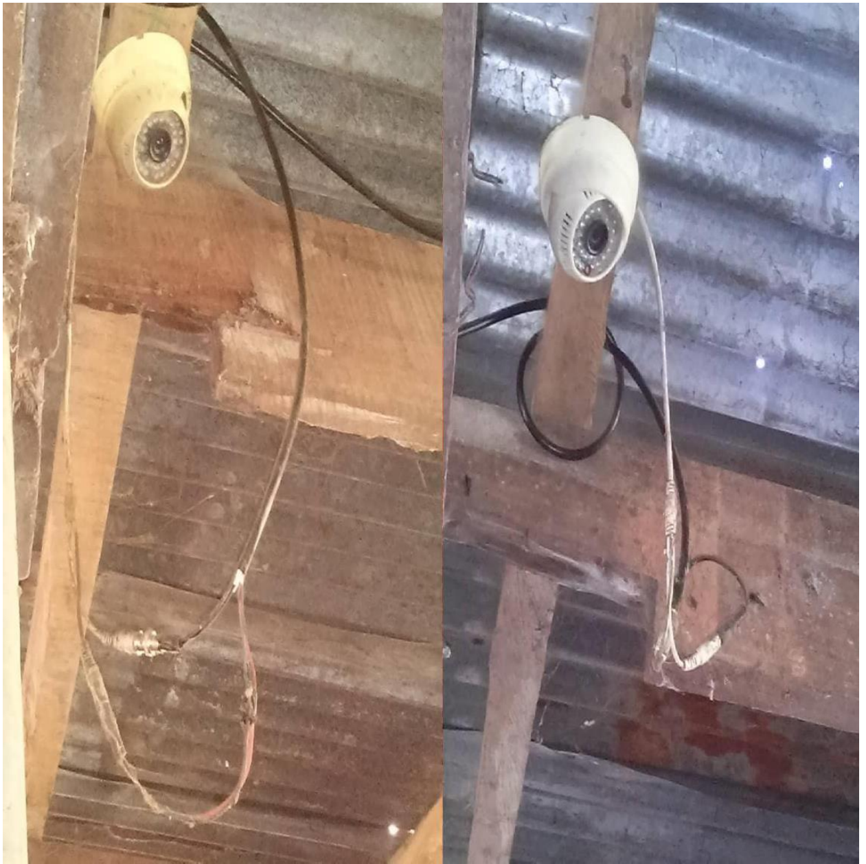
Plate 3.1. Cross- section of some of the installed Close circuit televisions (CCTV) used for behavioural recordings of experimental animals during the studies
