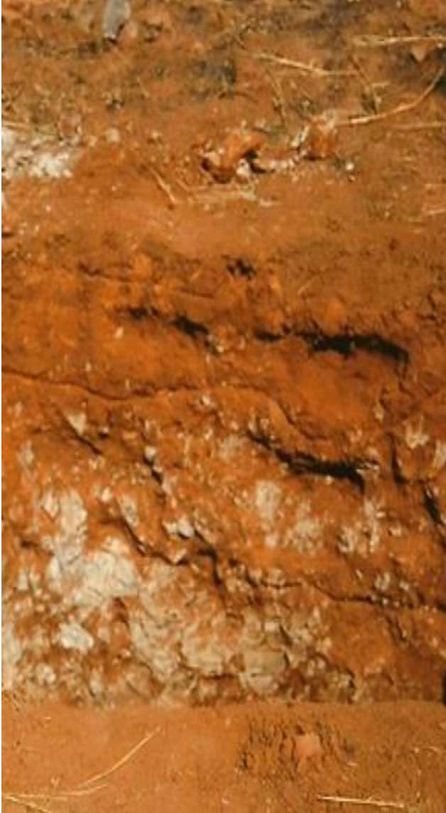
Plate 4.6: Profile Pit JP-BST-1, at the crest of toposequence (JP-BST1) of soils derived from Basalt, in Riyom, on the Jos Plateau, Nigeria (Parent material encountered at the depth of 82 cm).
