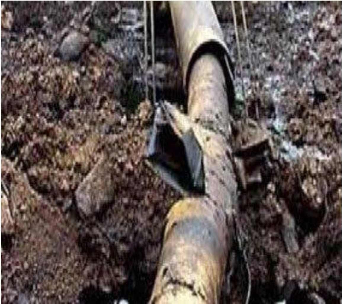
Plate 1.2: NNPC Vandalised pipeline in Forcados, Burutu LGA, Delta State, Nigeria
