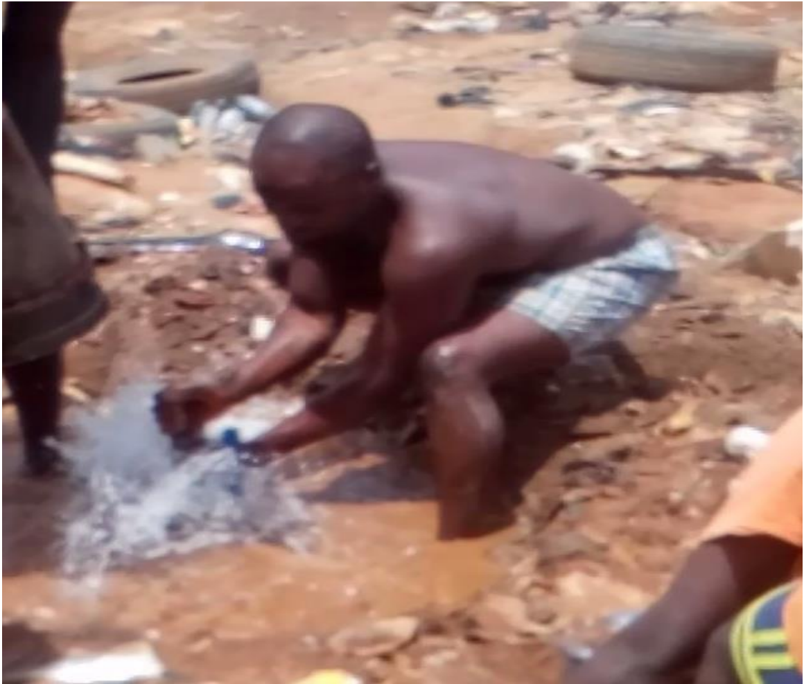
Plate 4.1 Repairs of vandalized pipe at Lagos by NNPC Engineers Source: field work (2018)
