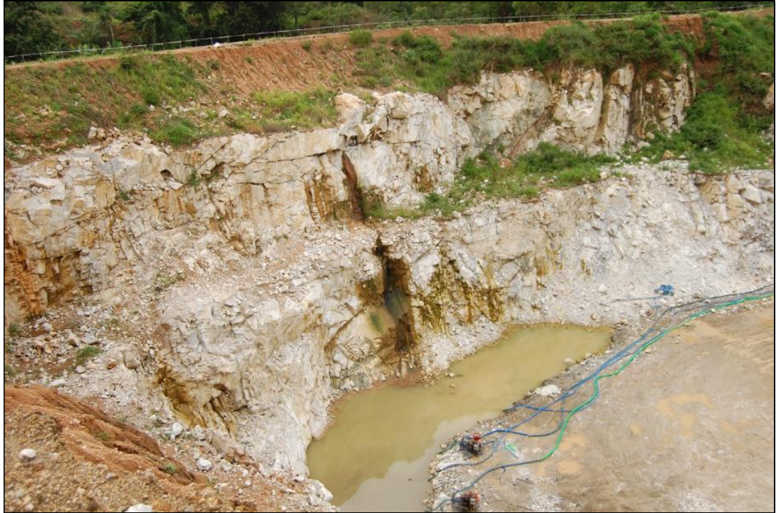
Figure 4.37: Pit Slope Picture Illustrating the Water Leakage Through Fractures
