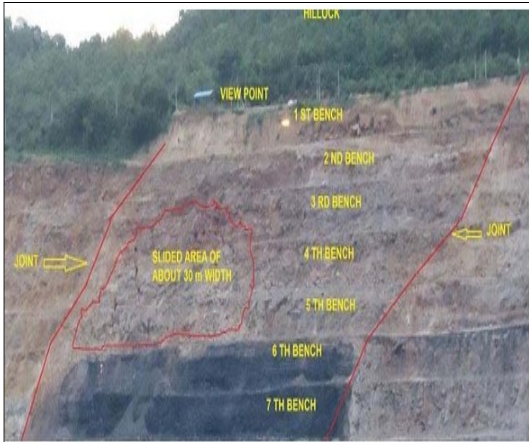
Figure 2.11: Slope Failure at Dorli Opencast project I (After Satyanarayana and Sinha, 2018)
