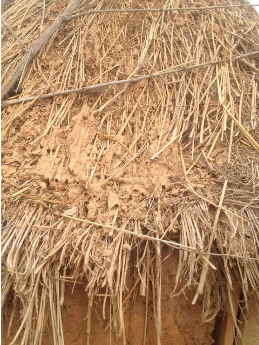
Plate 25: A Roof Infested by Termites (Fieldwork, Awe, 2017)
