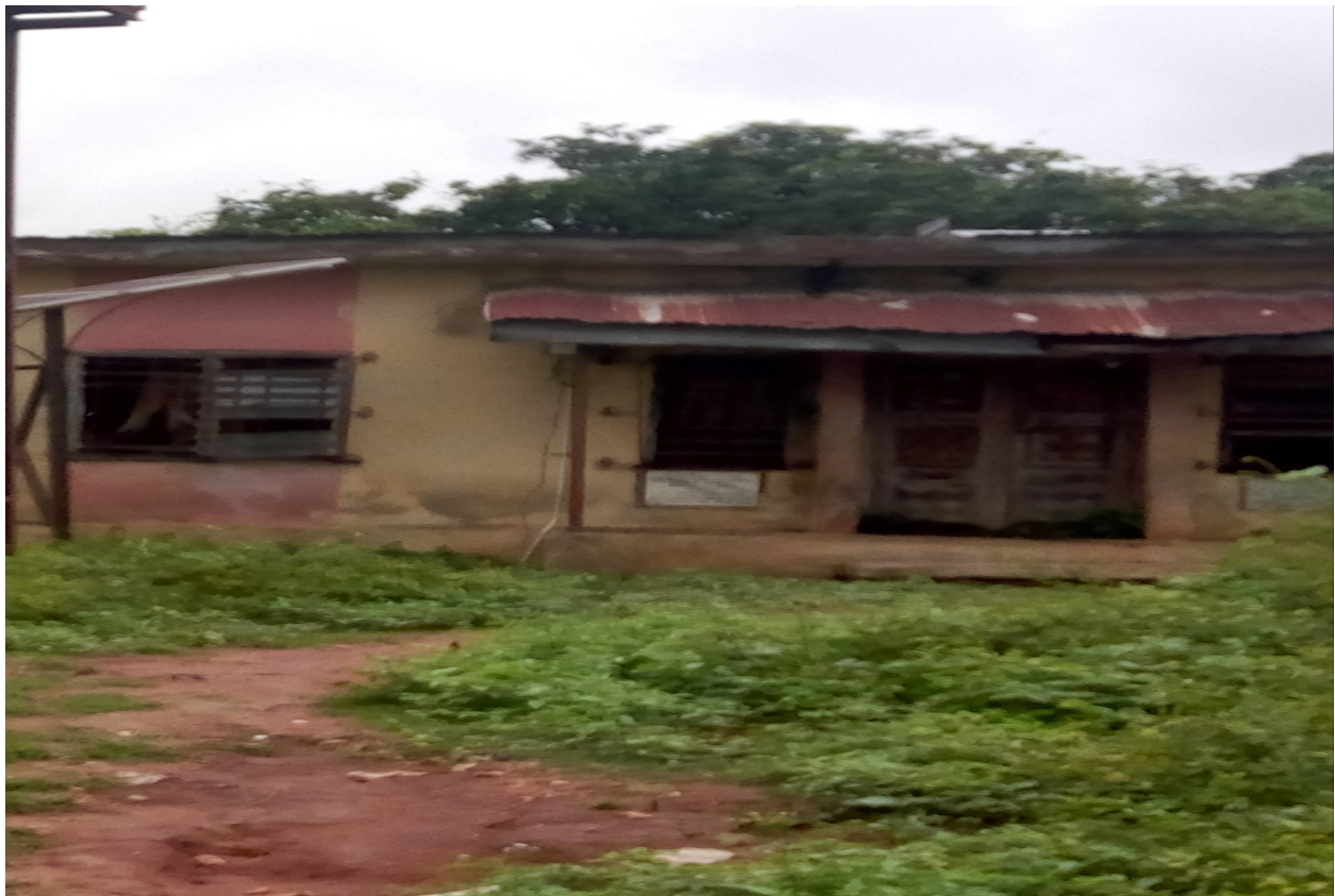
Plate 5: A picture showing a dilapidated health facility infrastructural condition in one of the rural communities sampled
