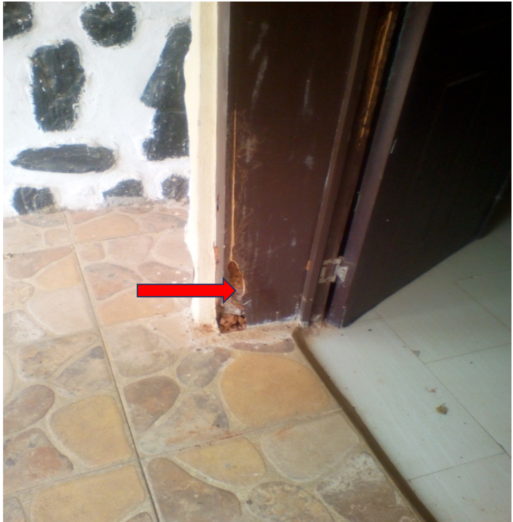
Plate 6: Dilapidation at Ikogosi Warm Spring Resort: Conference room door attacked by termite
