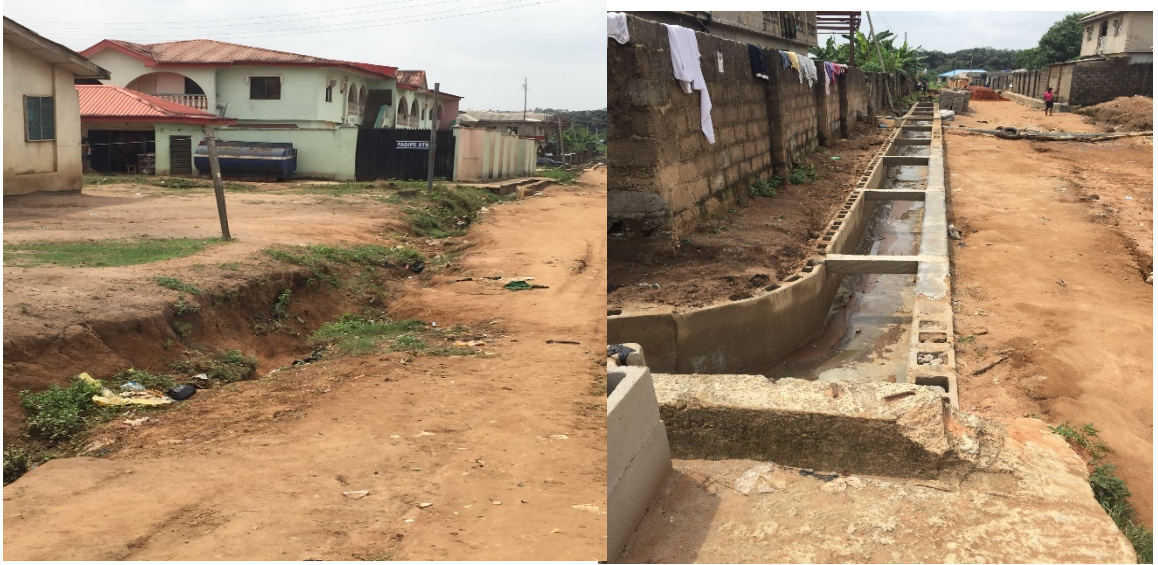
PLATE 7.3: Common Internal Road / Drainage condition in the study area: Fadipe Street Igando Source: Field survey, 2016
