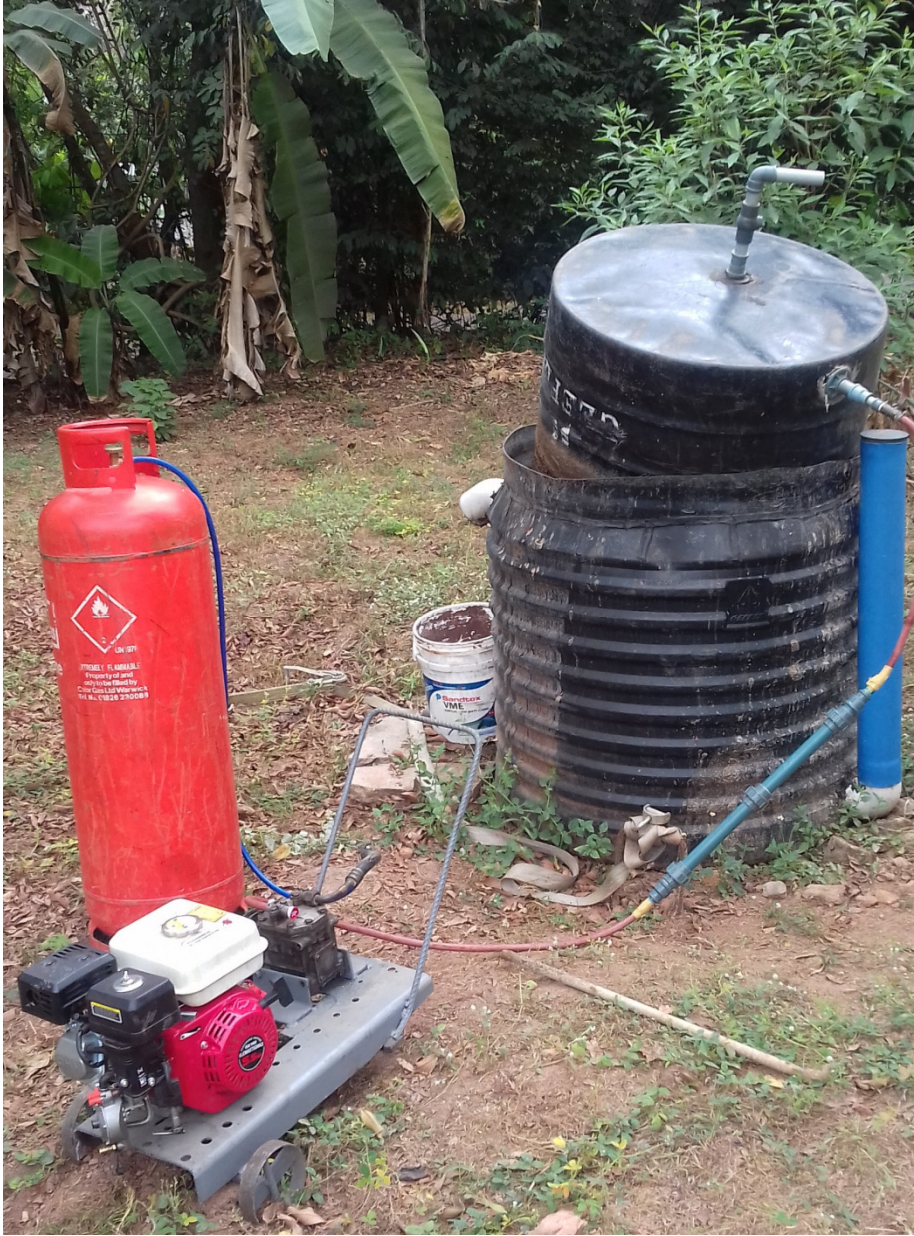
Set up for harvesting raw Biogas into cylinder
